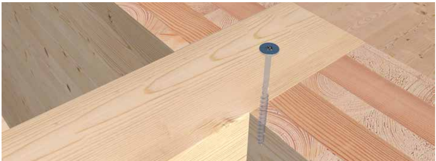
A downstand beam is fastened to the notched CLT wall by means of the SawTec partially threaded screw.
